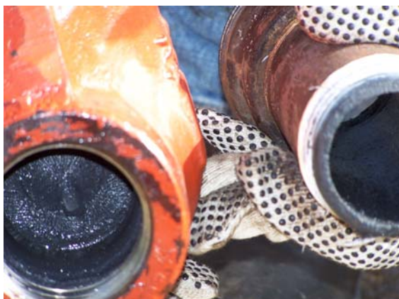
Figure 13 Inlet and discharge of check valve clear of scale after 8 months
